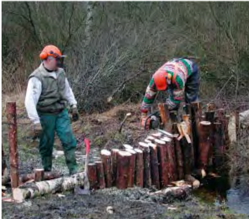
Construction of a dam. In Germany, more than 30 dams were built in order to restore the hydrology of the Kulz peat bog in north-eastern Bavaria, by closing off streams draining the bog. The water level was raised everywhere in the bog, and the new hydrological conditions should render the bog active again (© Photo Verein zum Schutz wertvoller Landschaftsbestandteile in der Oberpfalz e.V).
