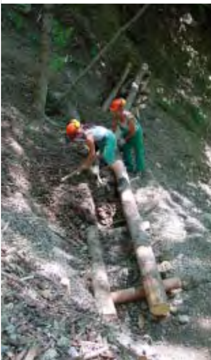
Laying a path to stabilise a slope in Italy. (© Photo Azienda Regionale delle Foreste).
